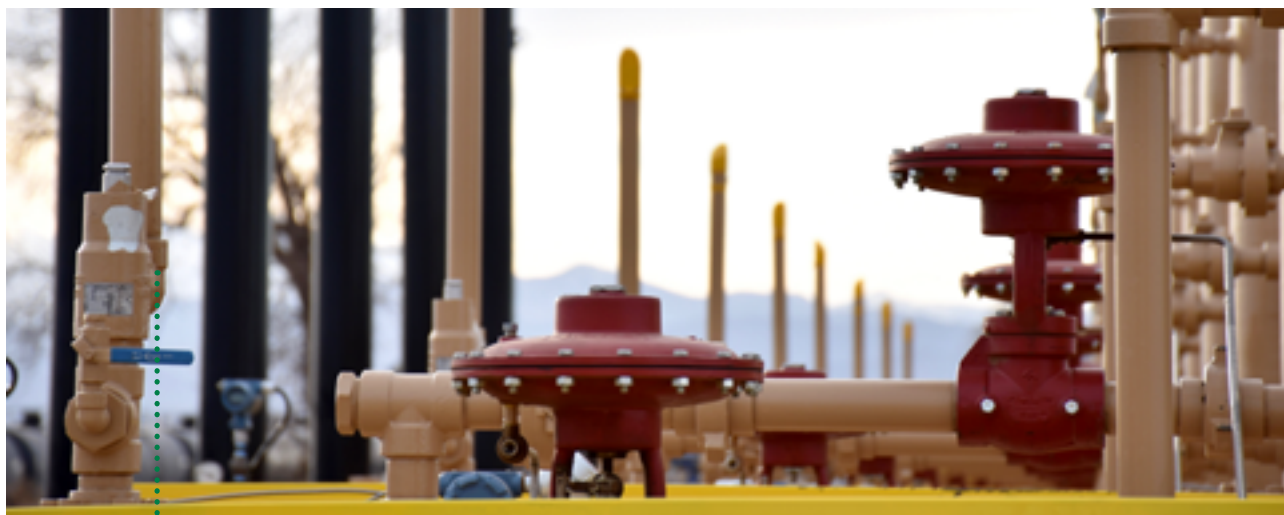
• A PLANT FOR THE SEPARATION OF OIL, GAS AND WATER IN COLORADO
